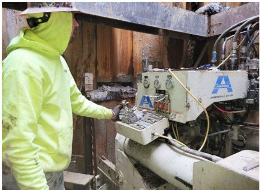
Jacking shaft was a compact 13 feet – one-meter pipe lengths were used for installation
