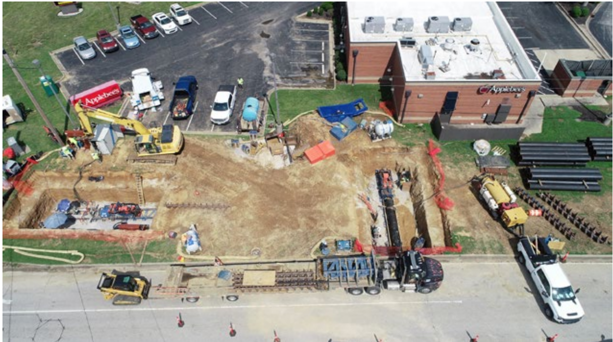
Projects such as the one shown above is an example of how contractors, such as Snyder Construction of Evansville, IN, utilize their Akkerman 240A GBM system. Snyder Construction was able to use one GBM system to accurately install pilot tubes and keep two auger boring machines productive, while minimizing disturbance to the public
