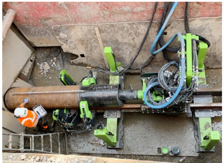
Technician uses the remote control to operate the GEONEX HZR610 drill machine set up for 10-foot casing lengths
